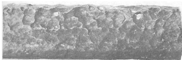
98.140 Figure 12-12.—General fireside thinning of a stainless steel superheater tube (results of fuel ash damage).
